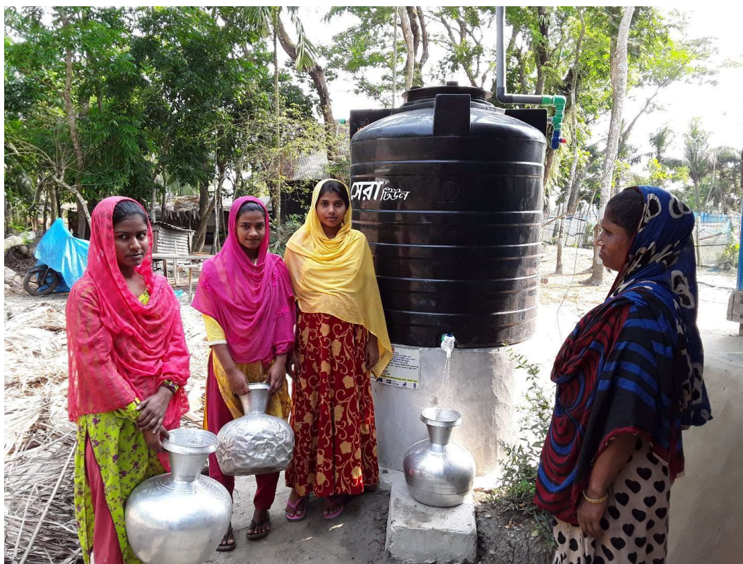
Figure 41 - Rainwater harvesting systems
