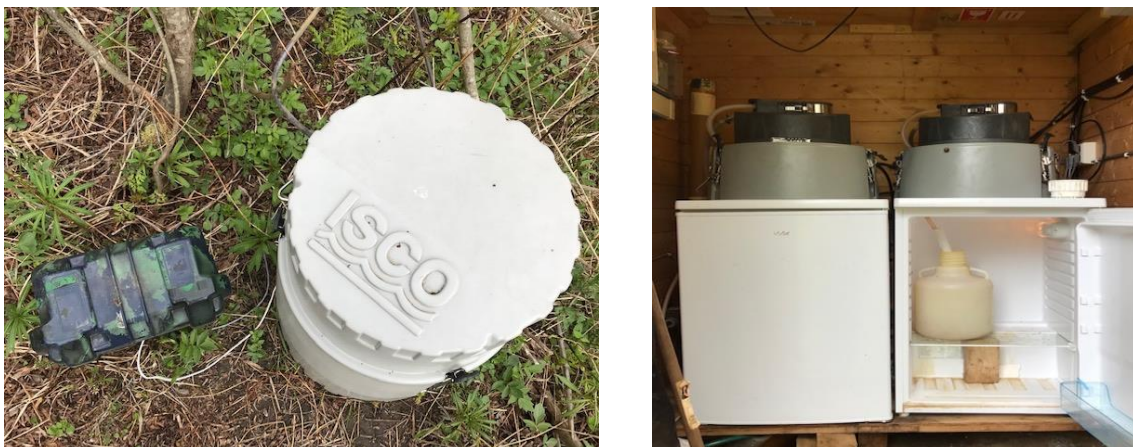
Figure 3.3: To the left: The portable automatic sampler at the inlet connected to a car battery for power supply. To the right: The automatic sampler at the outlet connected to a refrigerator. The outlet sampler is inside the sampling house. (Pictures taken 05.05.22).
