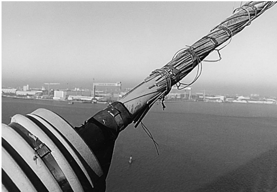
Figure 2 Saint-Nazaire cable failure [3]
