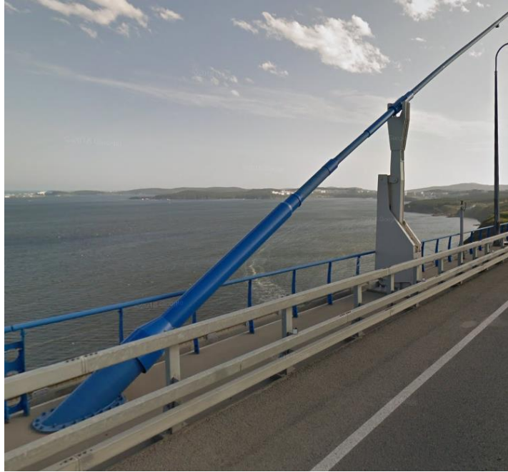
Figure 22 Russky bridge damper [15]
