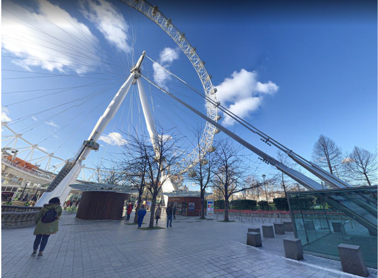
Figure 71 Back stay of London Eye featuring a Stockbridge damper [15]
