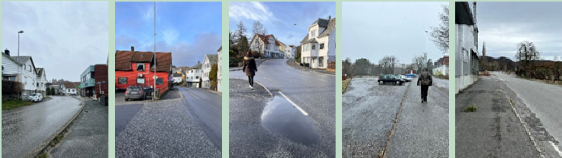
Figure 25: Showing pathways characterized with uneven road level, broken paths, and unclear segregation marks Source: Own Photo
