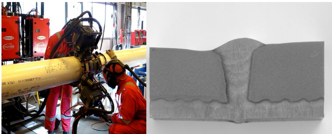
Figure 8-2 Mechanized PGMAW in operation and typical girth weld showing CMT weld roots (Karunakaran et al., 2013)
