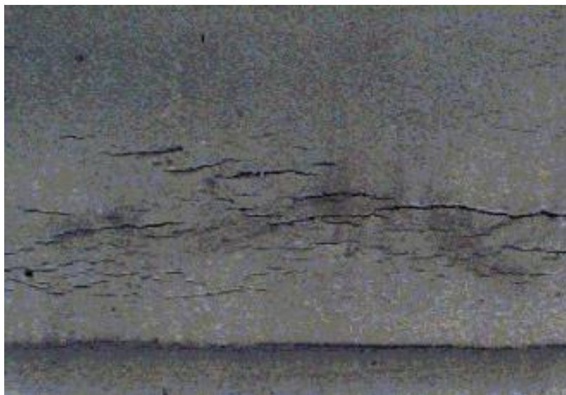
Figure 2-5 - Pipeline crack (Goedecke, et al., 2014)
