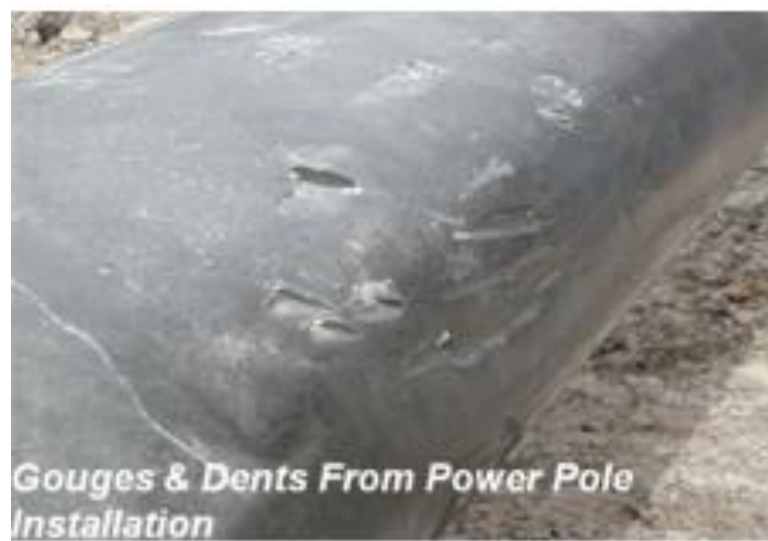
Figure 2-4 – Gouges in a pipeline (wolverinepipeline, 2010)
