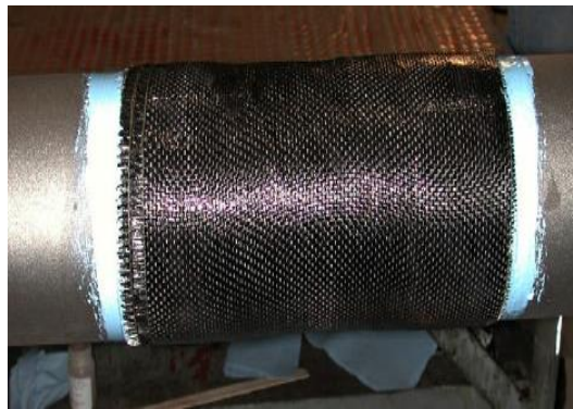
Figure 2-11 - Repaired test pipe with epoxy putty and carbon fiber wrapping (Duell, et al., 2008)
