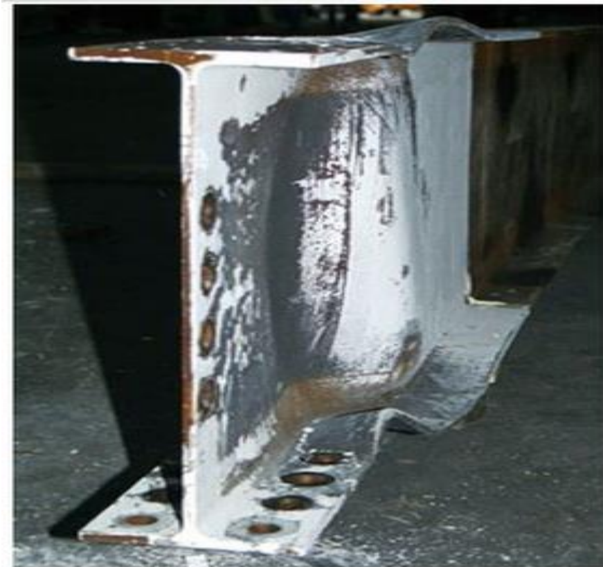
Fig. 2.3.1- Failure of beam due to buckling
