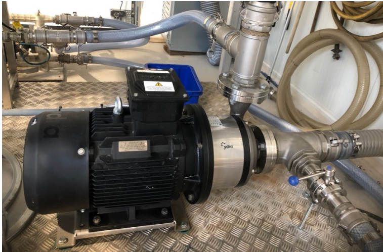
Figure 5: The centrifugal pump at the NORCE mixing unit
