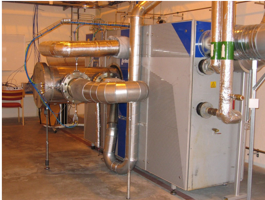
Figure 2. The MGT test rig.
