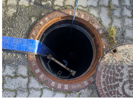
(b) Pump cable from manhole of tank 3
