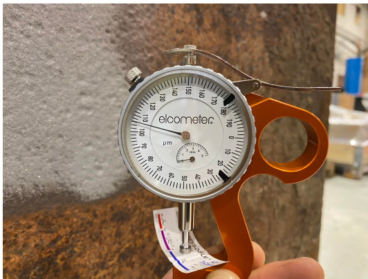
Figure 11: Surface Profile: Rust Flaked Surface
