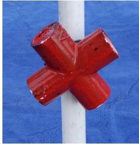
(a) Biological material on structure
