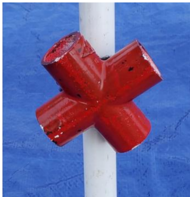
(a) Biological material on structure
