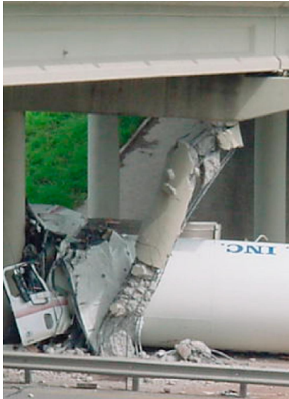
Figur 9: Fullstendig søylesvikt (V.DO, Pham, & Hao, Dynamic responses and failure modes of bridge columns under vehicle collision, 2018)
