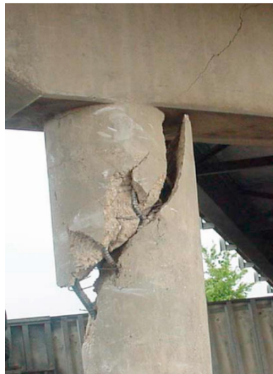
Figur 8: Skjærsvikt på søyle (V.DO, Pham, & Hao, Dynamic responses and failure modes of bridge columns under vehicle collision, 2018)
