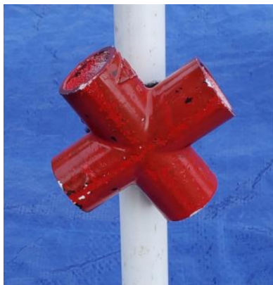
(a) Biological material on structure
