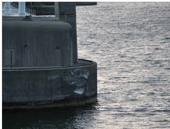
Figure 4.9: Ship Collision at Nordhordland Bridge in 2009 [15].
