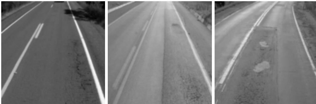
Figure 5.1: Images of roads with cracks
