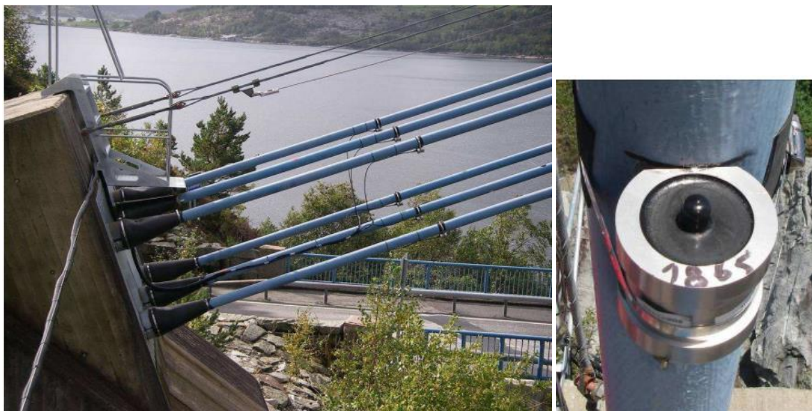
Figure 11 Acoustic sensor assembly details on the backstay cables
