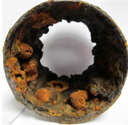
Figure 13: Formation of microorganisms in pipelines [57]
