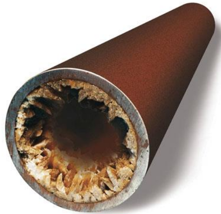
Figure 12: Formation of scale in pipeline [55]
