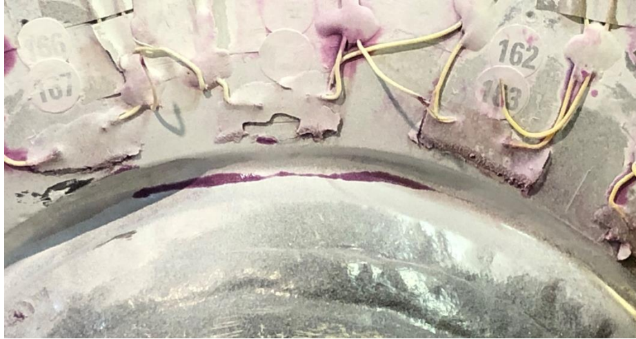
Figure 6-29: Quadrant Q1 repair, material removal by grinding to achieve shorter crack length.
