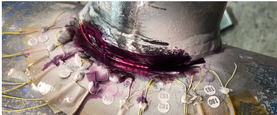
Figure 6-27: Quadrant Q3 repair, crack removal by grinding, dye penetrant application. Specimen DT4.
