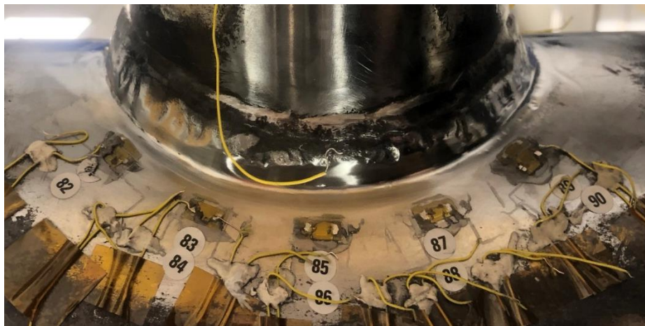
Figure 6-14: Quadrant Q4 repair: crack removal by grinding at the centre of the saddle and weld toe improvement by grinding all the quadrant.
