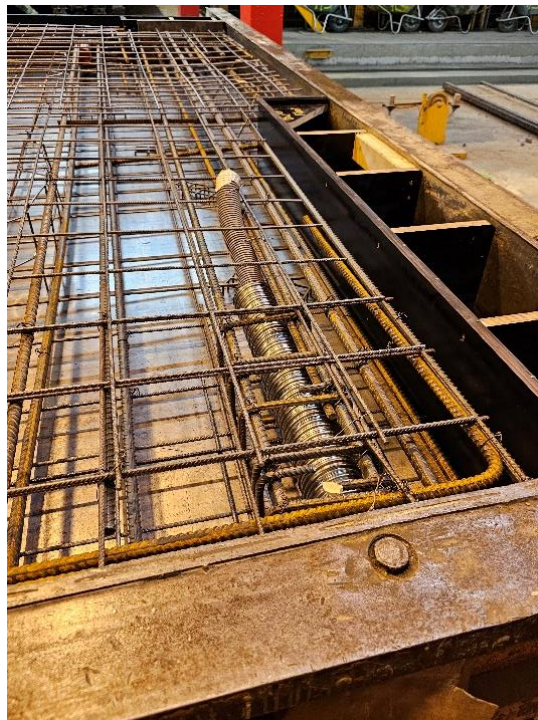
Figure 29: Mould used by Veidekke Prefab for use of conduit in precast concrete elements. Taken 05.02.2024
