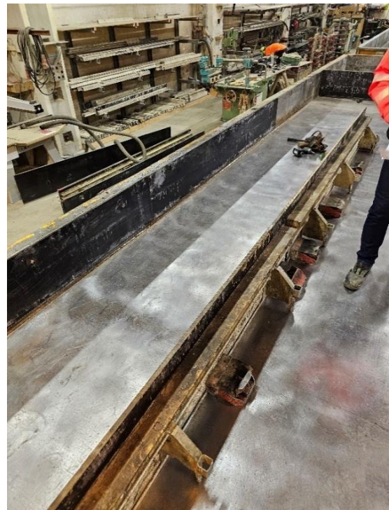
Figure 6: Wooden panels with magnetic fasteners are placed to customize the shape of the element. Taken on 05.02.2024, at Klepp
