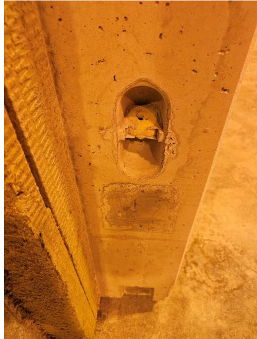
Figure 19: Close up of lifting handles for concrete slab, stored at Veidekke Prefab. Taken on 05.02.2024, at Klepp
