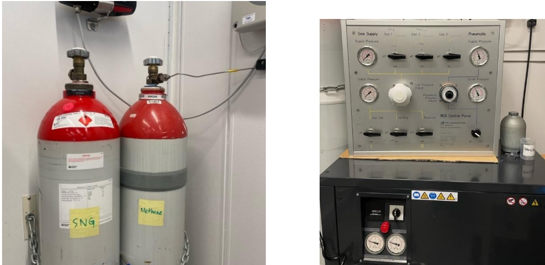
Figure 3.6 SNG and methane gas bottles, and "Gas Supply" box and compressor.
