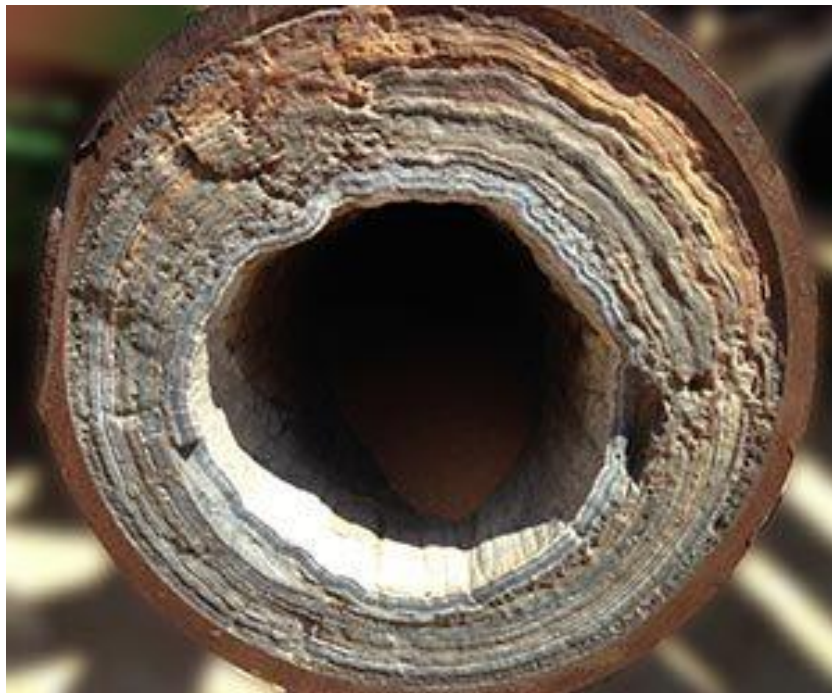
Figure 3.1 Barium sulfate scale in production pipe [16].
