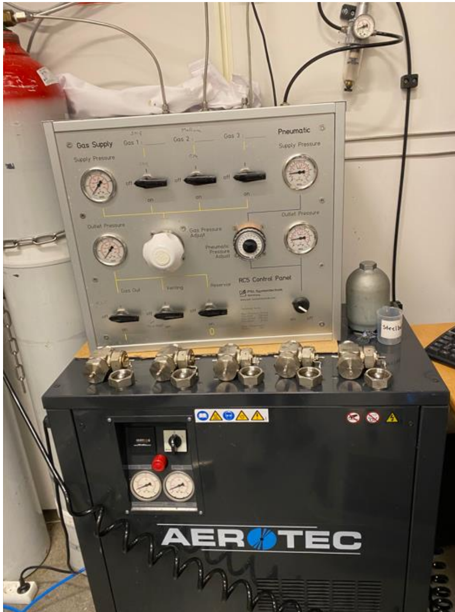
Figure 2.5 SNG bottle, RC-Control Panel box, and compressor unit. The five cells used for testing are on top of the compressor.
