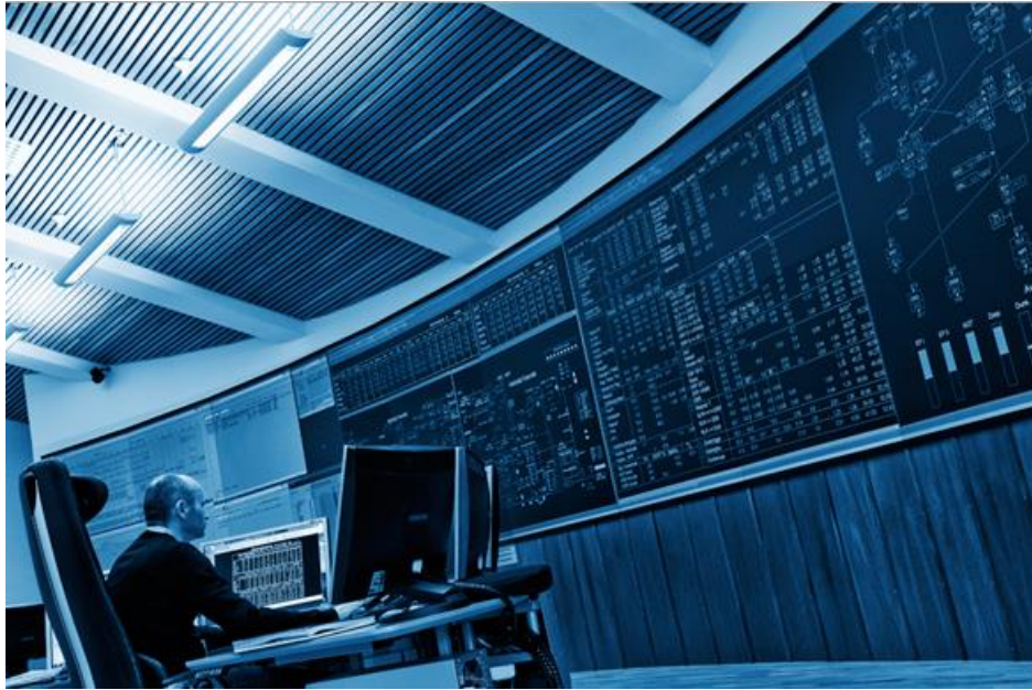
Figure 2: Gassco’s control room at Karmøy, Norway (Gassco, n.d.)
